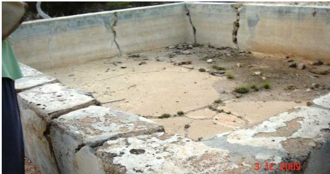
Broken water reservoirs Dabis River (GWX)
