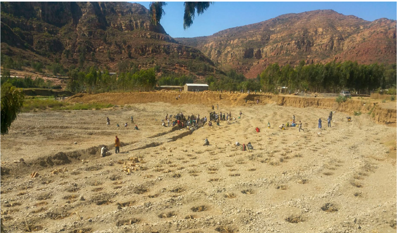
Converting a big gully or river valley at Gergera watershed through innovative reclamation practices. Photo by Niguse Hagazi (ICRAF)
